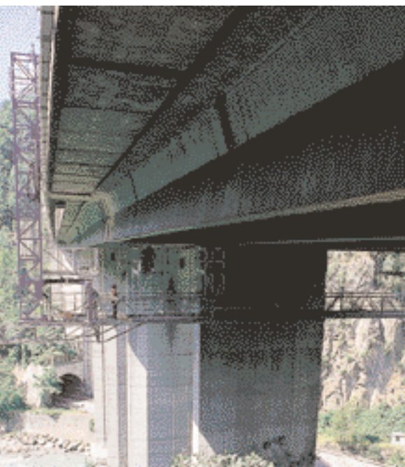
Since some of the piers are very tall, work on the underside will be done from mobile retractable platforms.
