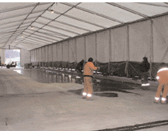
Work on the upper surface will be done under a mobile tunnel moving along rails as the work progresses.
