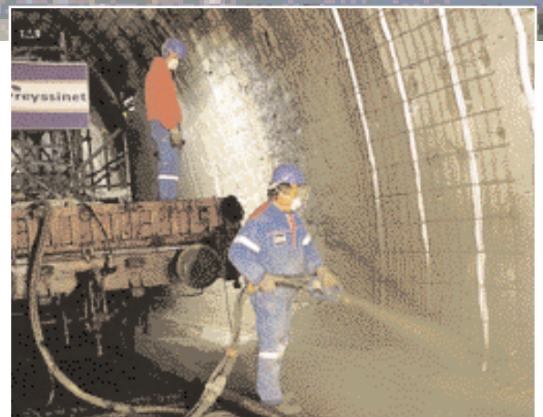
Freyssinet has strengthened the Fix-St-Geney's tunnel in France by installing a 12 cm thick shotcrete ring.
